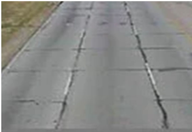
Joint Reflection Cracking
